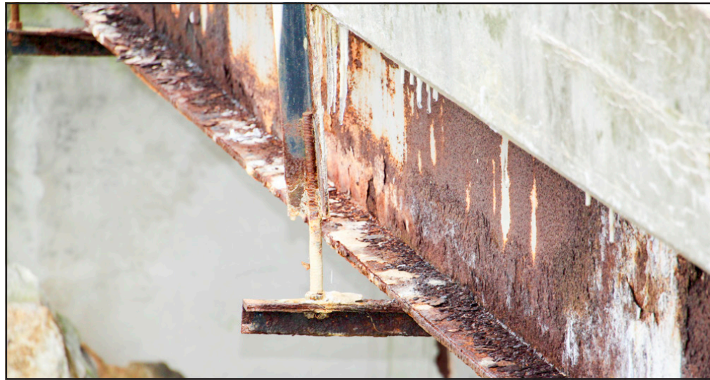
The Fisher Field Road bridge is suffering from extensive corrosion and is in the process of being replaced. Photo by Shawn Jarrard
