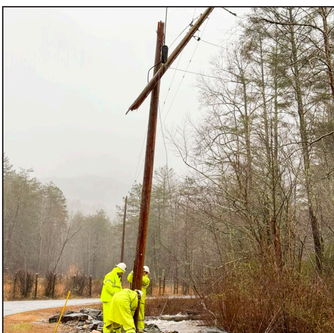
Blue Ridge Mountain EMC linemen were able to get power up and running within 24 hours for customers who lost electricity due to the storm early last week. Photo/Facebook students.
